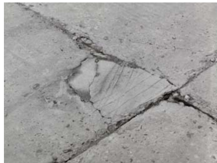
Primary source of FOD- Pavement debris
